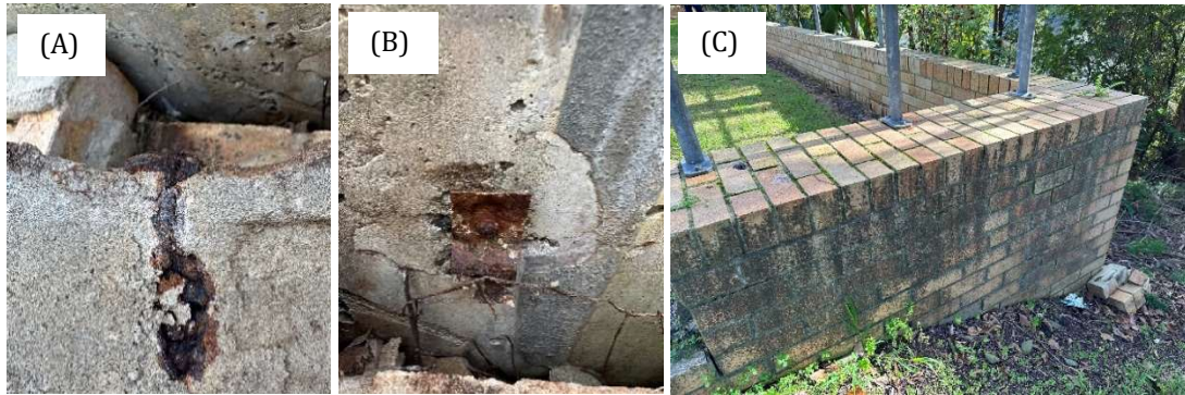
FIGURE 5: 40-YEAR-OLD BRICK VENEER RETAINING WALL AT SITE IN WYOMING, NSW WITH EXAMPLE OF BRICK TIE CORROSION (A) WITHIN MORTAR, (B) ACHORED TO CONCRETE WALL AND (C) THE CONDITION OF THE WALL OVERALL
