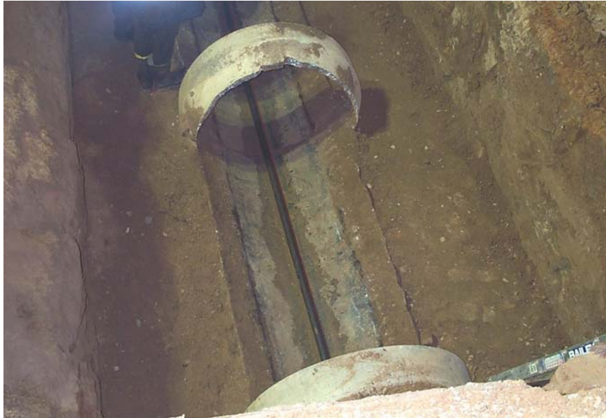
Figure A7 - Relining of a corroded reinforced concrete sewer pipes shows the crown of the pipe has been severely corroded leaving only the base of the pipe and the collars at the joints where they were provided with some protection by the spigot of the other pipe.
