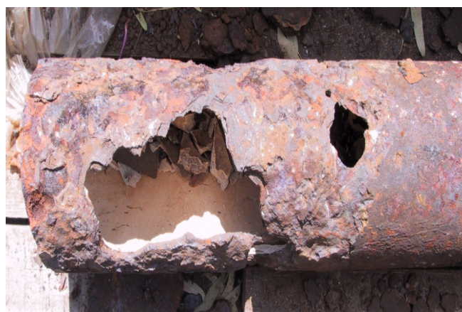
Figure A2 External corrosion of cast iron pipe
