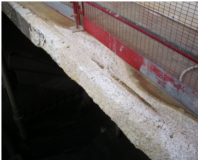
Figure A8 - Severe corrosion of concrete in an aeration tank covered to reduce odours. The corrosion was up to 75mm in 3- 4 years despite the use of an extraction system.
