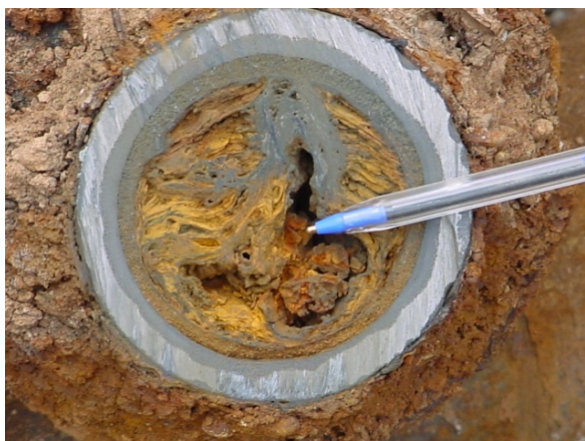
Figure A1 Internal corrosion of an unlined cast iron pipe
