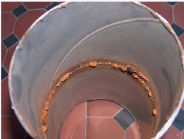
Fig 17: corrosion on untreated circ. weld but not on pickled spiral weld
