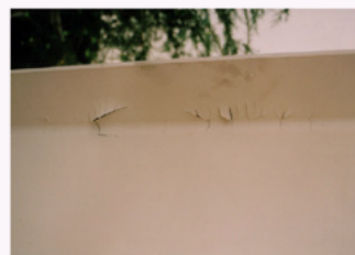
Fig 20A: Blistering in thick coating zones
