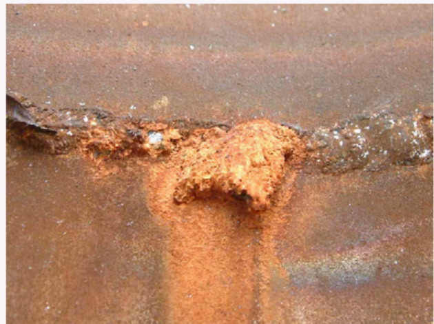
Fig 18: Corrosion of circ. Weld in 316 tank with raw water - note rainbow heat tint (Boulton, Nickel Institute)
