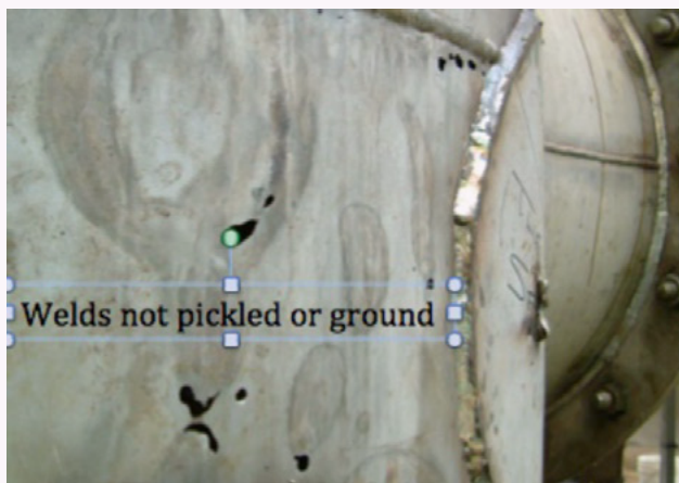
Figure 6A: Exterior of perforated scrubber vessel
