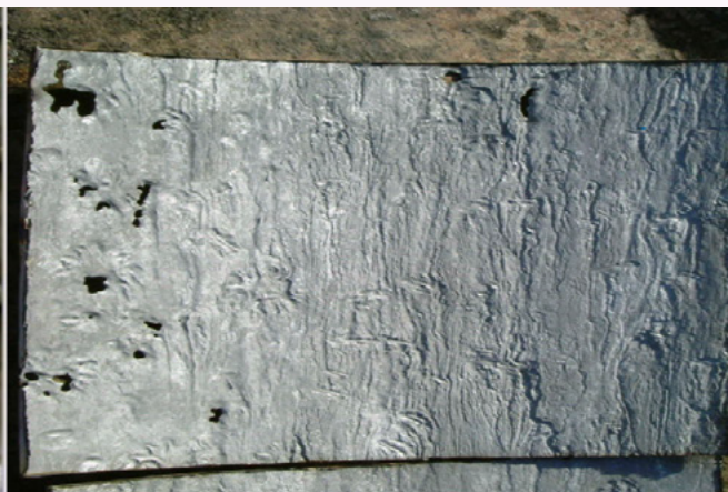
Figure 6B: Interior of discarded tank with perforations and erosion markings
