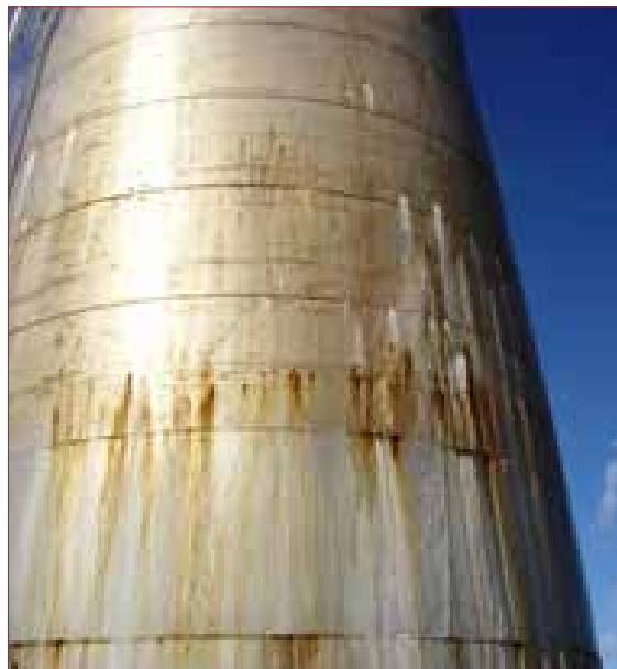
Stainless steel water tank weld corrosion leading to tank failure.
