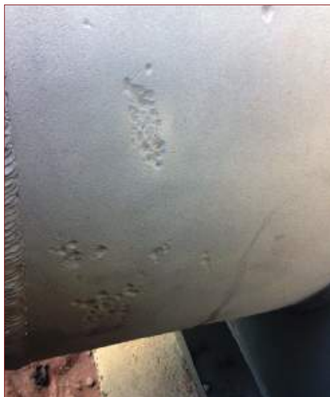
East End Corrosion.
