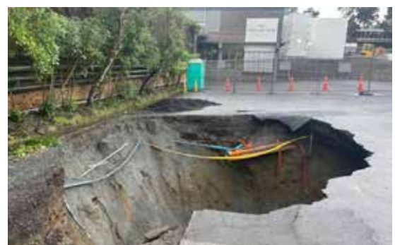
Below: The 2023 sinkhole in Parnell, Auckland
