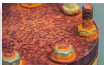
Metal connections and fasteners are susceptible to corrosion in salt air
